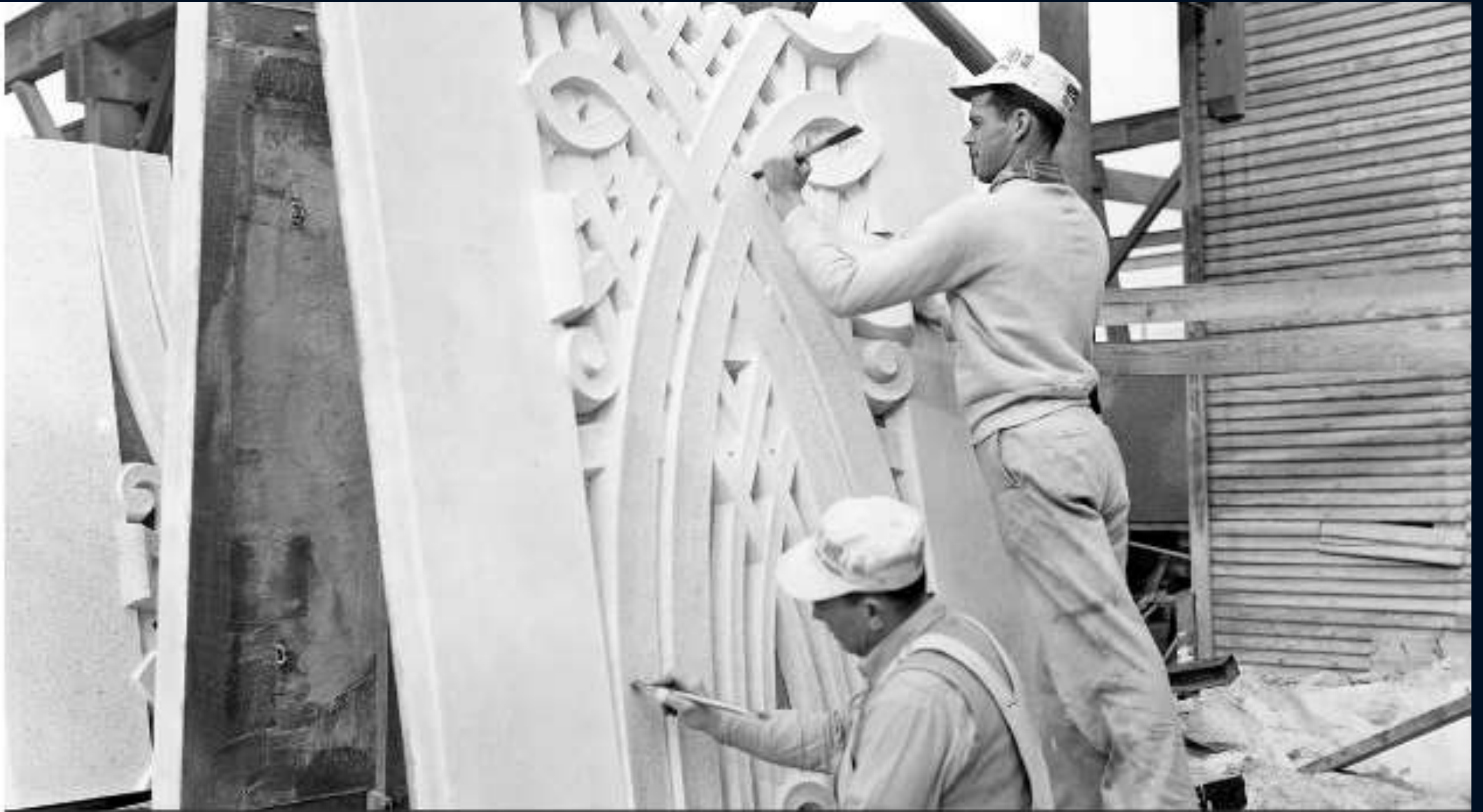
The concrete panels were cast in Virginia and shipped by railway car to the Temple site where workers attached them to the superstructure. (Photo from 1933).
