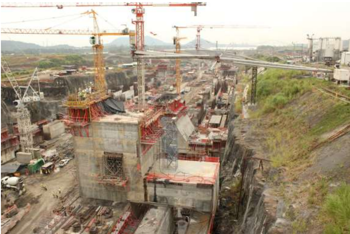
Gru e tower belts
